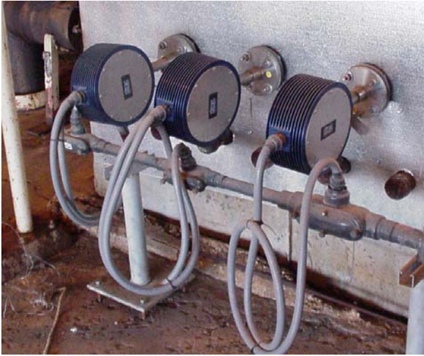
Figure A-5. Flex sensor connection for service loop, TA version using Liquid Tight Conduit.
